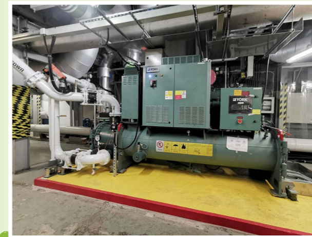
High efficiency night load chiller
